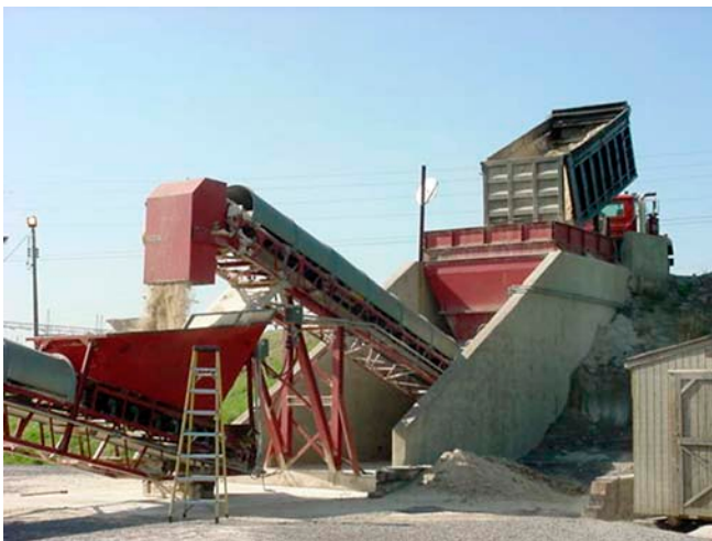
Figure 7-6. A covered conveyor distributes FGD gypsum at transfer points. (Miller, 2007.)
